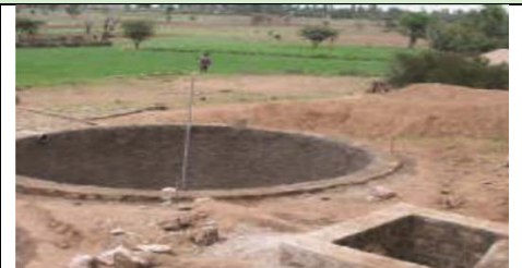
Figure 2.2.8. Partially constructed circular micro-pond with stone-lined walls and adjacent inlet/silt trap structure.
