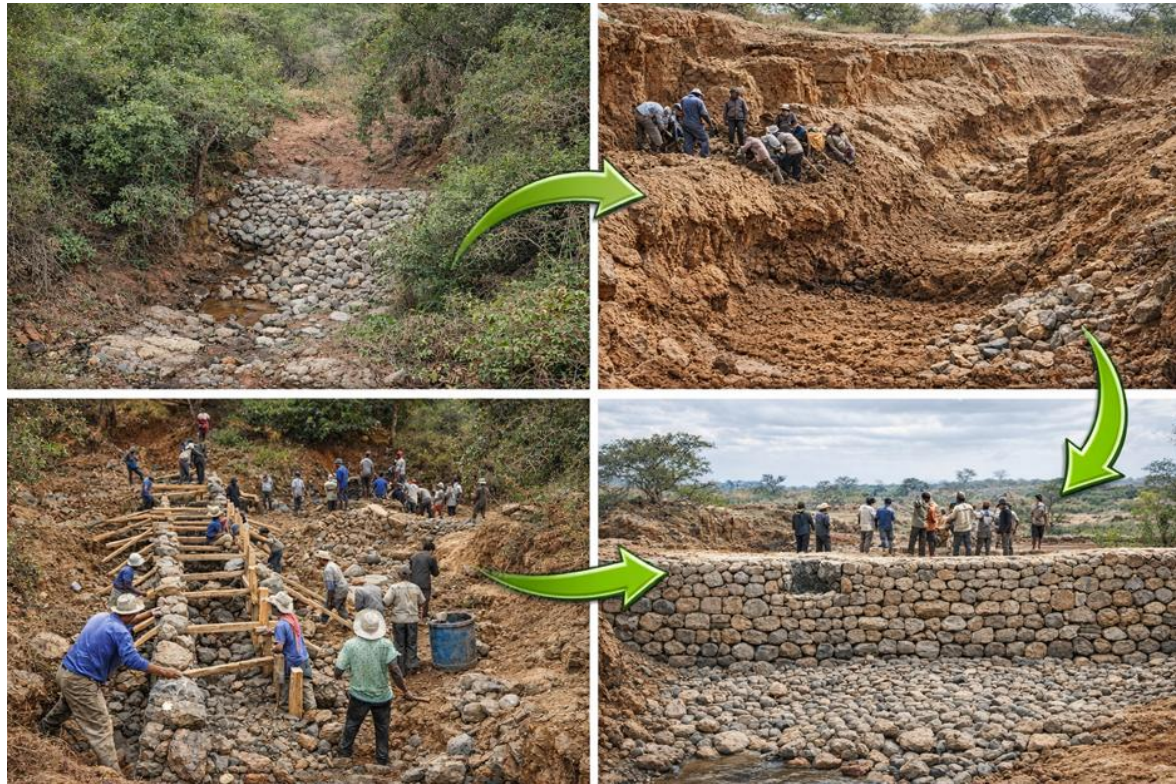
Figure 2.1.28. Step-by-step construction of a stone check dam showing excavation, stone placement, spillway shaping, and apron installation.
