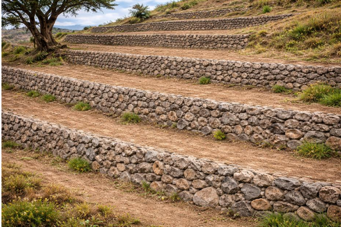
Figure 2.1.16. Stone bund constructed along contour lines to control runoff and enhance infiltration.
